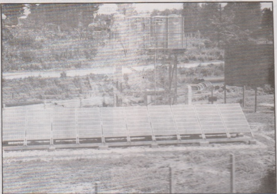
Fig. 11. Photovoltaic Water Pumping at Sundarighat, Kirtipur, Kathmandu (Nepal)
